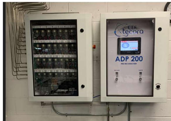
Example of installation : 32 ways instrument
